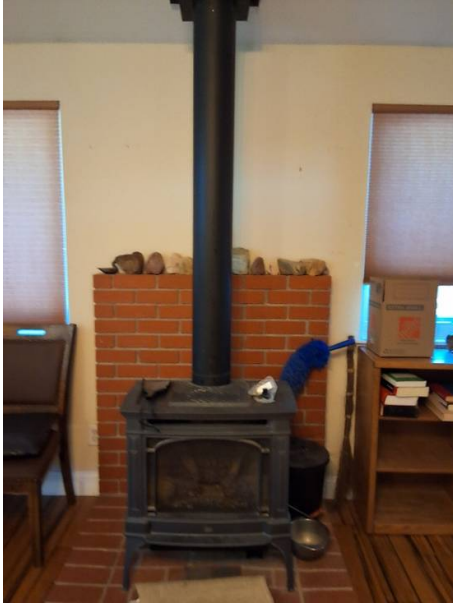
Gas fireplace in living room
