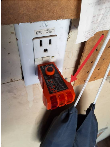
Garage outlet on South wall
