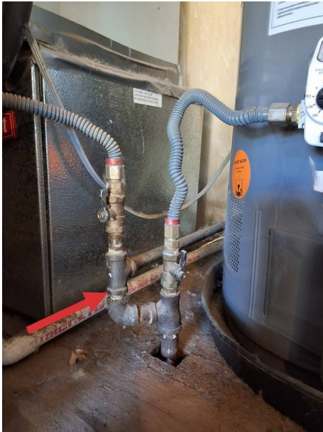
Gas supply line to forced air unit
