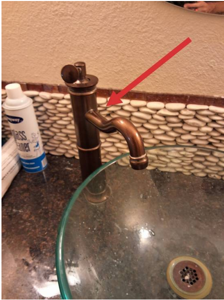
Loose faucet at hallway bathroom.
