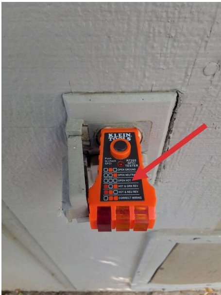
Outlet located outside, on rear of garage
