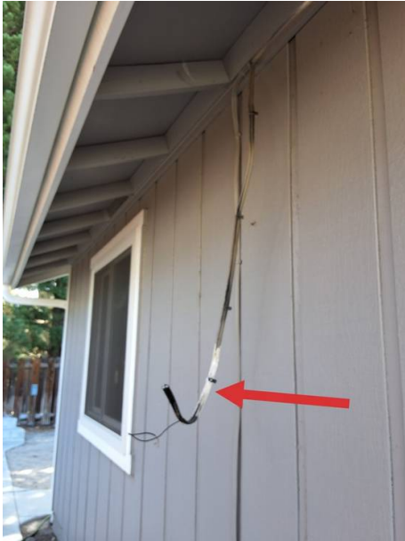
TV cable line at north of home
