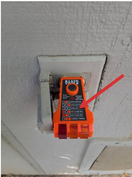
Outlet located outside, on rear of garage
