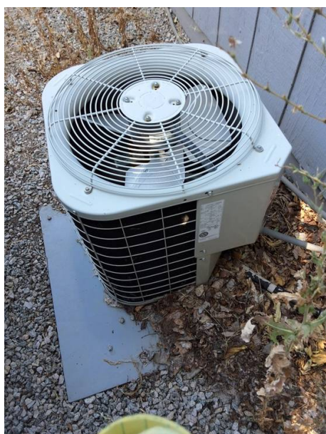
AC. unit on South side of home
