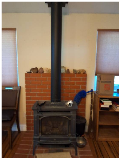
Gas fireplace in living room
