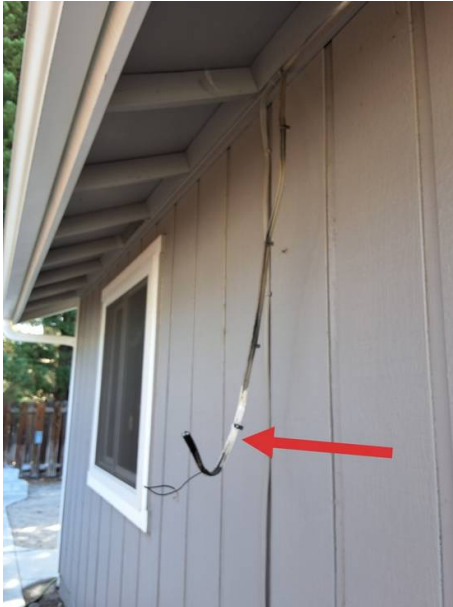
TV cable line at north of home
