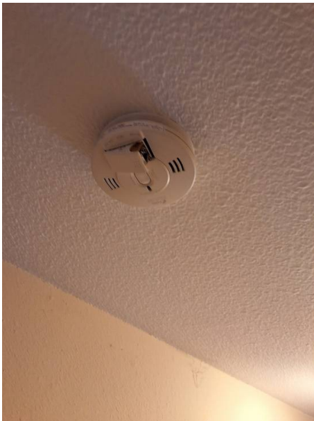
Smoke / Monoxide detector in hallway
