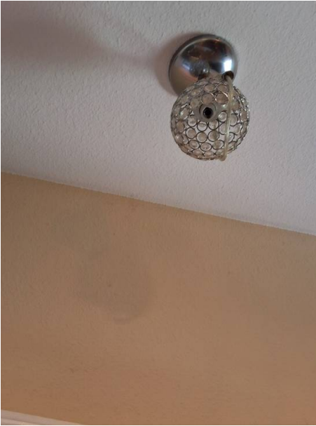
Light fixture over kitchen sink
