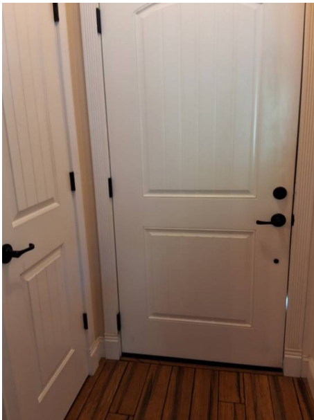
Missing door stops at entry and closet doors
