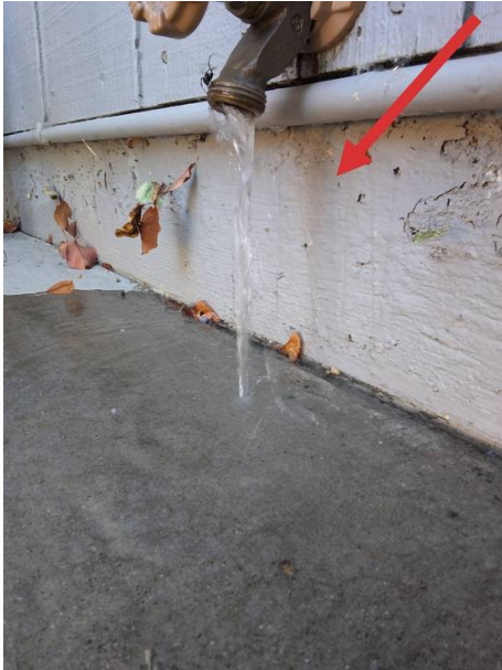
Hose bib at north side of home
