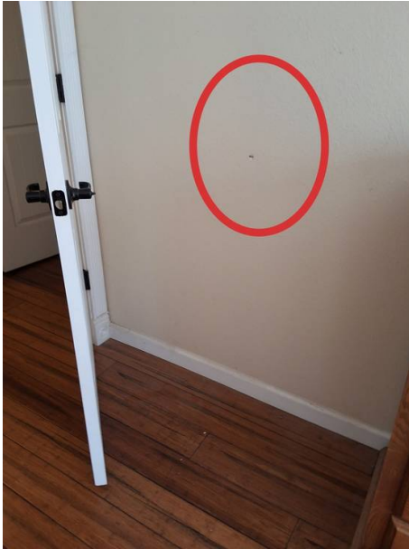
Wall damage due to non-present door stop in master bedroom
