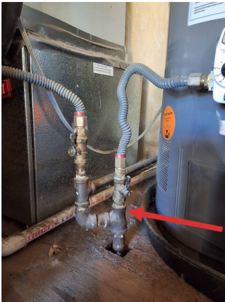
Gas supply line to water heater
