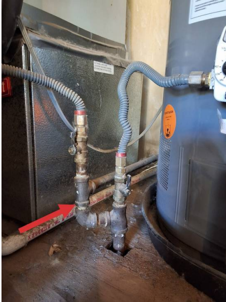
Gas supply line to forced air unit
