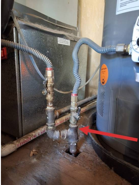
Gas supply line to water heater
