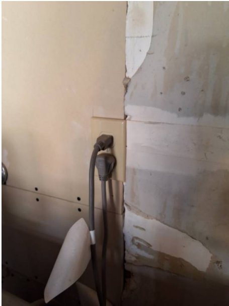
Non-GFCI outlet behind washer/dryer in garage
