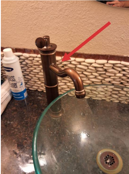
Loose faucet at hallway bathroom.
