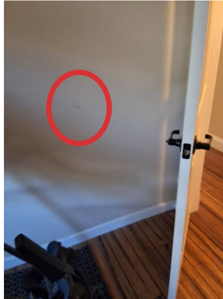
Wall damage due to non-present door stop in hallway bedroom
