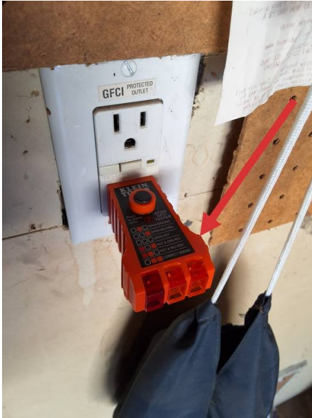
Garage outlet on South wall
