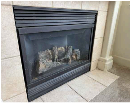
Gas Fireplaces: Wall Switch The gas fireplace responded to the wall switch and appeared functional.
