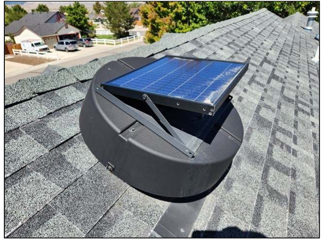
9.5 Item 2(Picture) Solar powered ventilation fan
