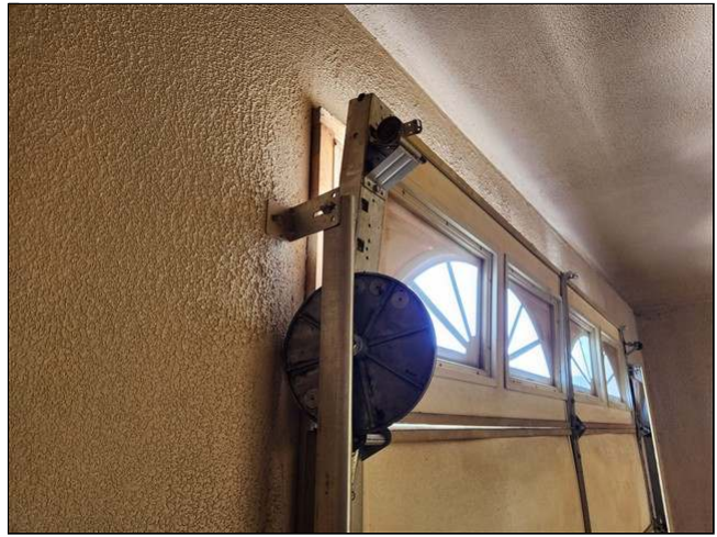
11.2 Item 2(Picture) Garage door is NOT fully installed
