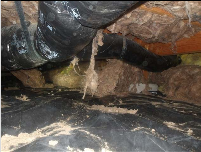
9.1 Item 2(Picture) fallen subfloor insulation
