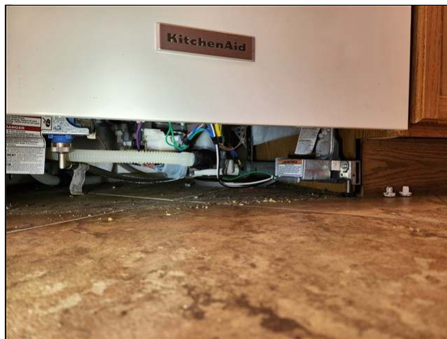
6.0 Item 2(Picture) dishwasher hookups
