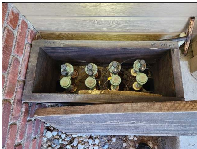
5.13 Item 2(Picture) irrigation box/valves
