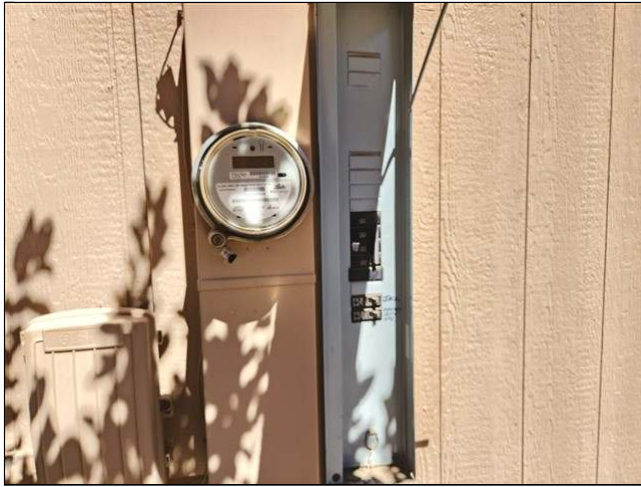
4.1 Item 3(Picture) main electrical panel
