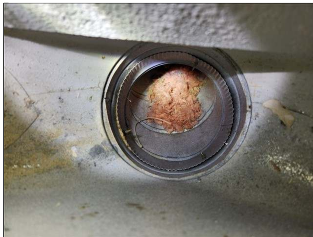
10.3 Item 2(Picture) debris (and mice nest/urine odor) seen in the vents
