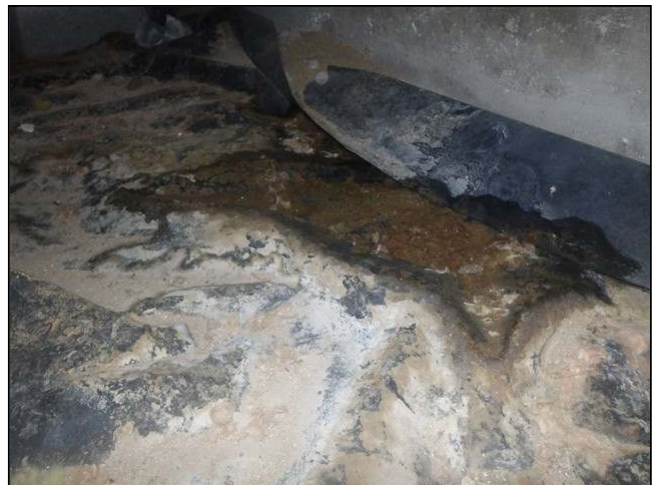
5.3 Item 4(Picture) moisture from leak
