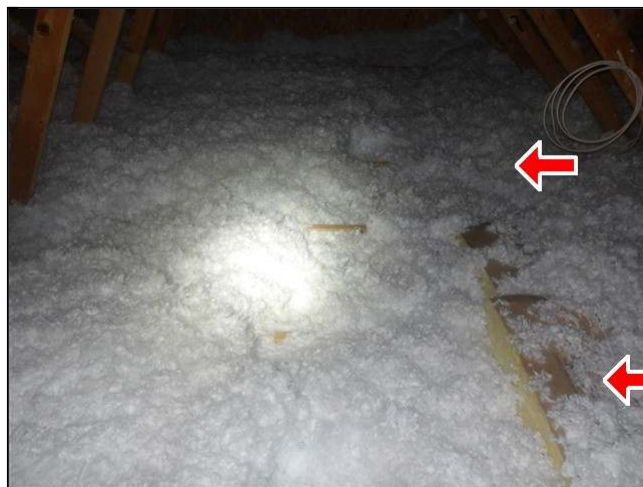
9.0 Item 2(Picture) tapering down to about R19 in a few locations
