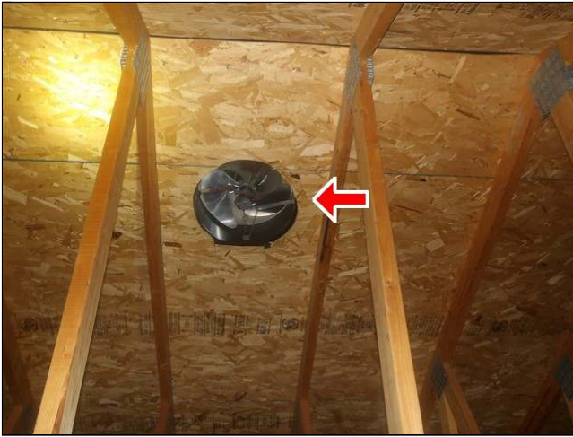
9.5 Item 1(Picture) Solar powered ventilation fan
