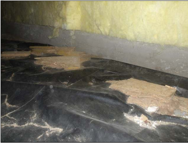
3.2 Item 1(Picture) Construction debris (and/or trash) should be removed
