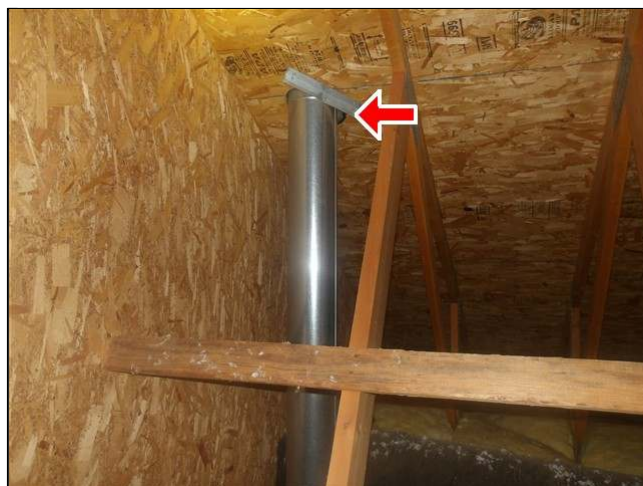
9.4 Item 2(Picture) properly ducted to the exterior
