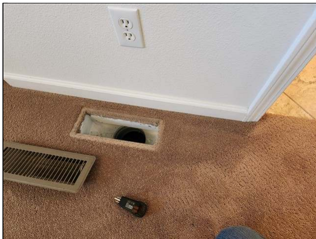
10.3 Item 1(Picture) debris (and mice nest/urine odor) seen in the vents
