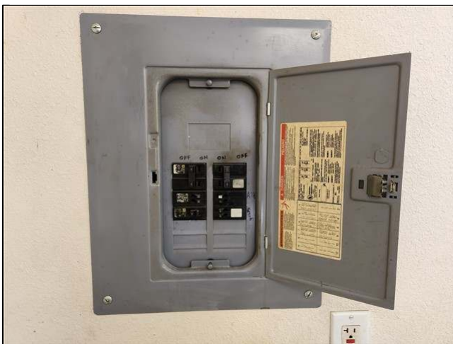
11.6 Item 1(Picture) main garage panel
