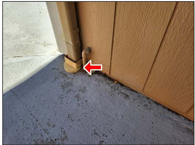
2.4 Item 2(Picture) in-ground drains for gutter downspouts
