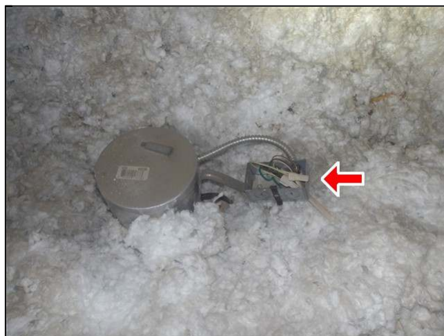
4.5 Item 3(Picture) Open wire connection
