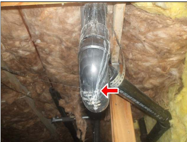
5.3 Item 3(Picture) master bath shower drain leaking
