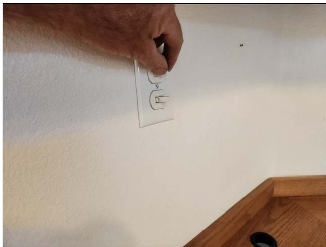
4.5 Item 1(Picture) Faulty light switch noted at the Office
