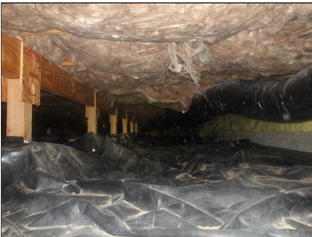
3.6 Item 1(Picture) due to subfloor insulation
