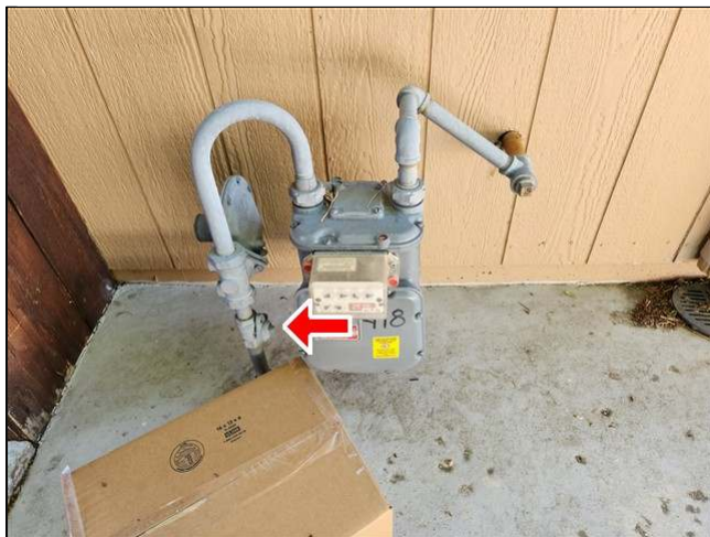
5.11 Item 1(Picture) main gas shut-off valve
