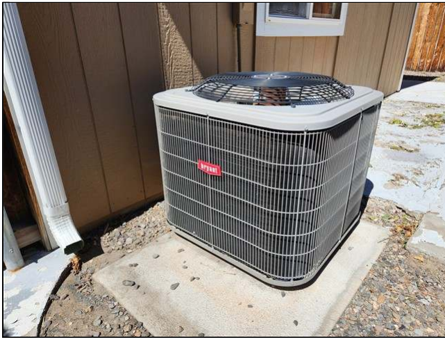
10.5 Item 1(Picture) condensing unit
