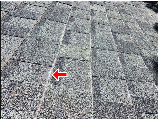
11.3 Item 3(Picture) Typical loss of granules noted
