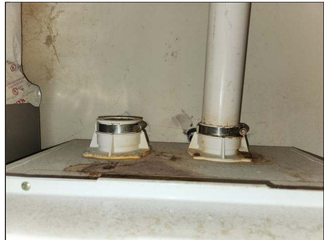
5.4 Item 4(Picture) combustion air and exhaust pipes
