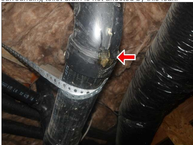
5.3 Item 5(Picture) guest bath toilet drain leak
