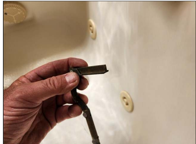
5.5 Item 2(Picture) drain plug broken
