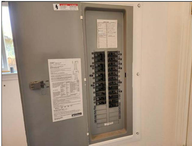
4.1 Item 1(Picture) laundry room panel
