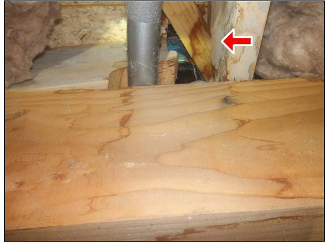
5.3 Item 2(Picture) master bath shower drain leaking
