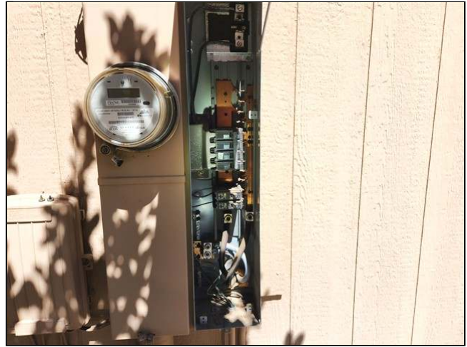
4.1 Item 4(Picture) main panel conductors
