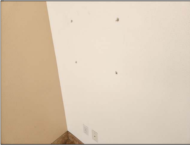
7.2 Item 1(Picture) Typical holes through drywall
