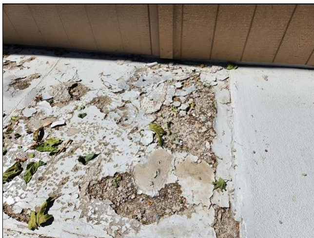
1.7 Item 1(Picture) Spalling damage of the concrete surfaces
