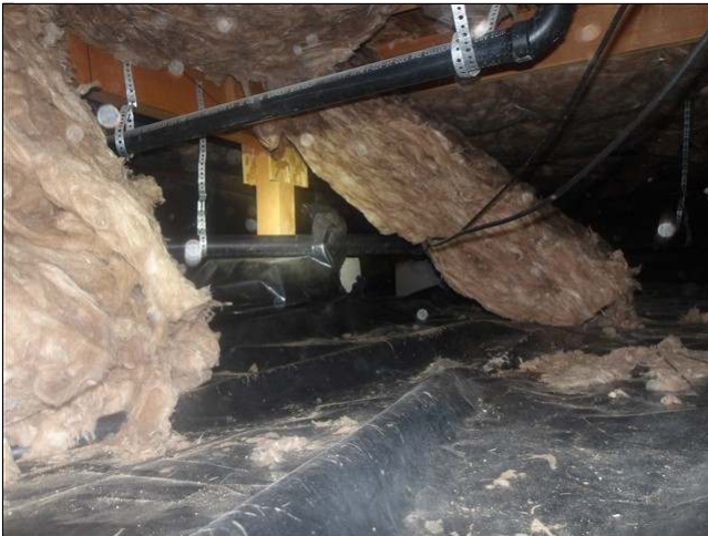
9.1 Item 4(Picture) fallen subfloor insulation
