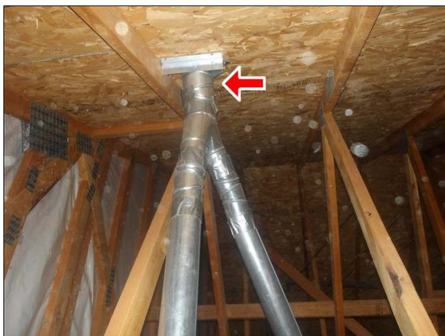
9.4 Item 1(Picture) properly ducted to the exterior
