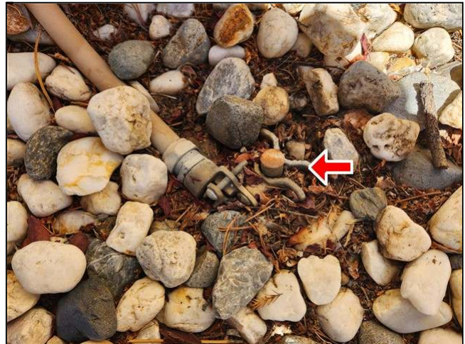
4.3 Item 2(Picture) grounding rod and clamp
