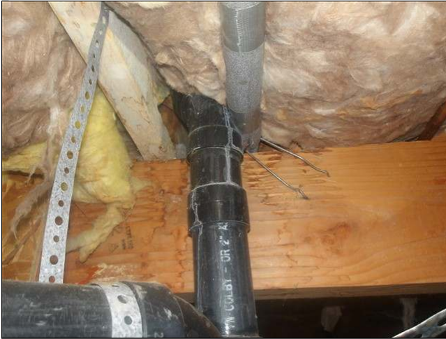
5.3 Item 1(Picture) master bath shower drain leaking
