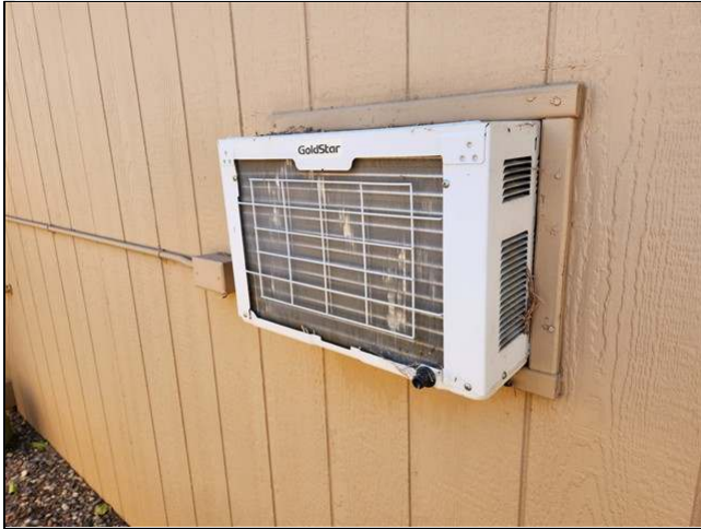
11.9 Item 1(Picture) cooling unit at north wall
