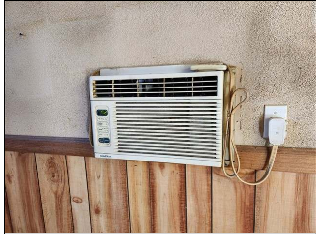
11.9 Item 2(Picture) cooling unit at north wall
