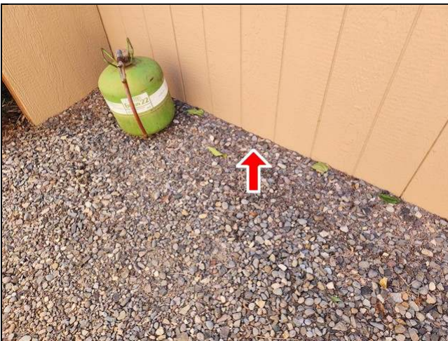
11.1 Item 5(Picture) Improper clearance under the lower edge of wall siding
