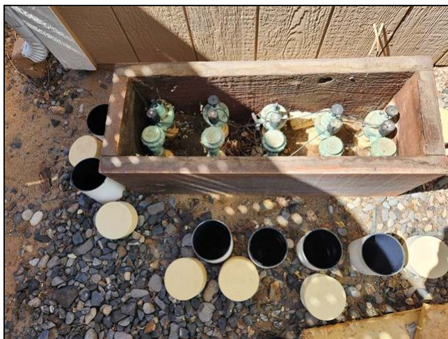
5.13 Item 1(Picture) irrigation box/valves
