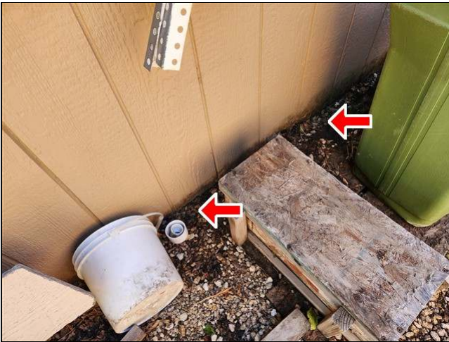
11.1 Item 3(Picture) Improper clearance under the lower edge of wall siding
