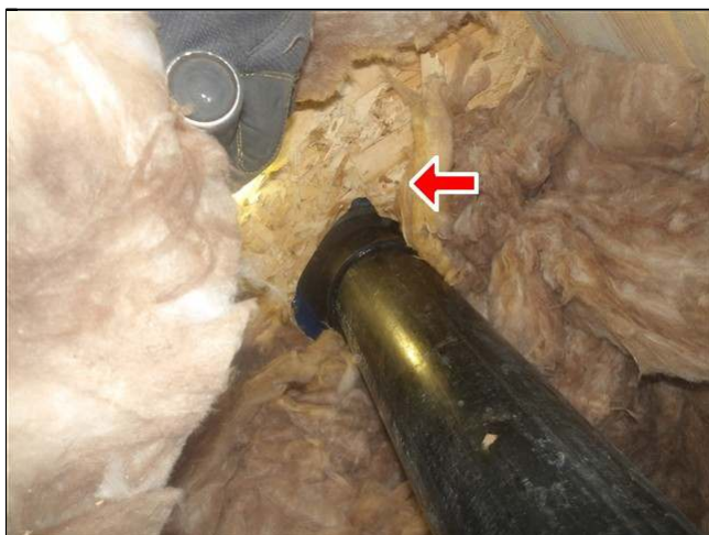
5.3 Item 7(Picture) subfloor not affected
