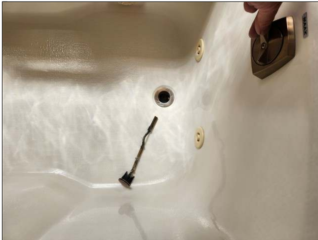
5.5 Item 1(Picture) drain plug broken
