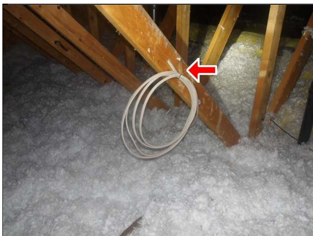
4.5 Item 2(Picture) loose wire end in attic area
