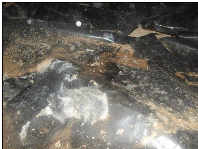
5.3 Item 6(Picture) moisture from leak
