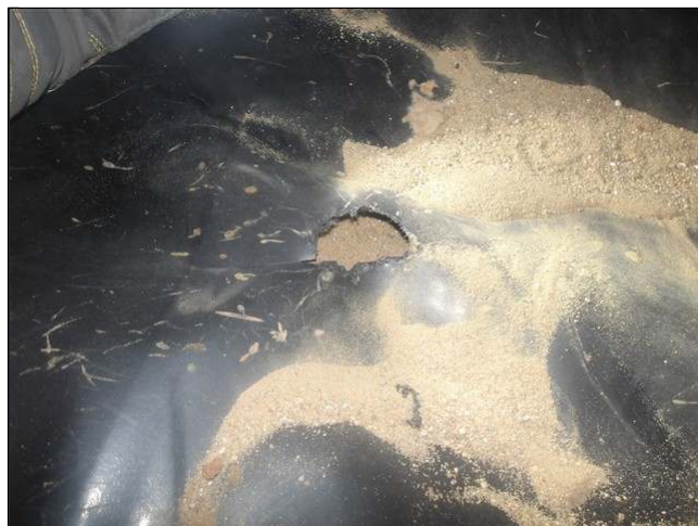
9.2 Item 2(Picture) rodent hole through vapor barrier
