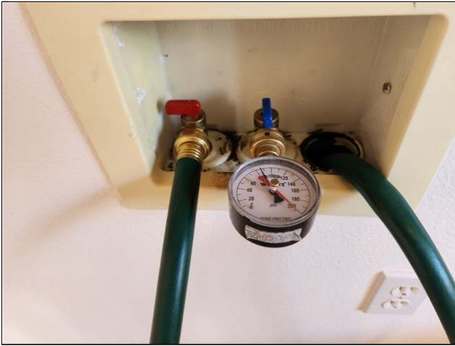
5.2 Item 1(Picture) water pressure at laundry connections
