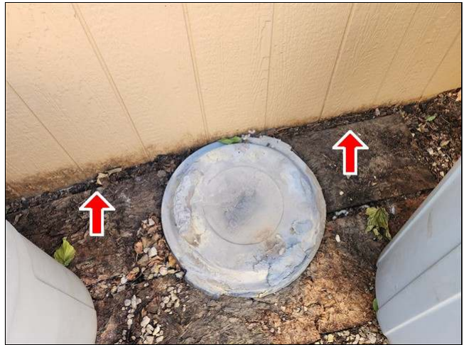
11.1 Item 4(Picture) Improper clearance under the lower edge of wall siding
