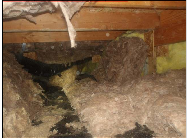
9.1 Item 3(Picture) fallen subfloor insulation
