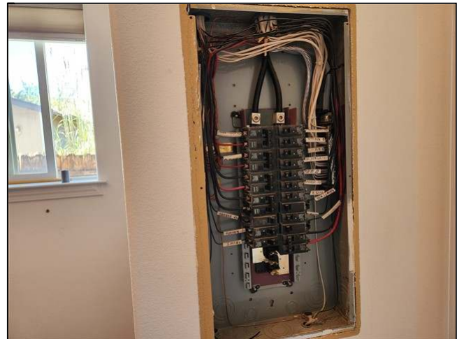
4.1 Item 2(Picture) panel conductors
