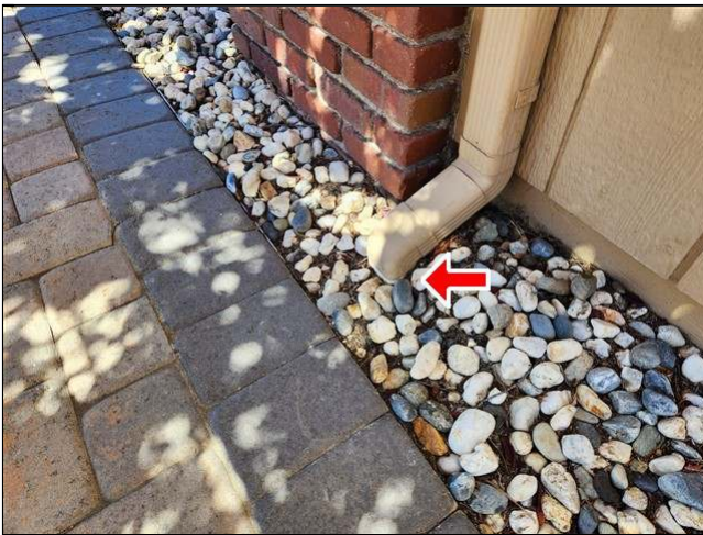
2.4 Item 1(Picture) in-ground drains for gutter downspouts
