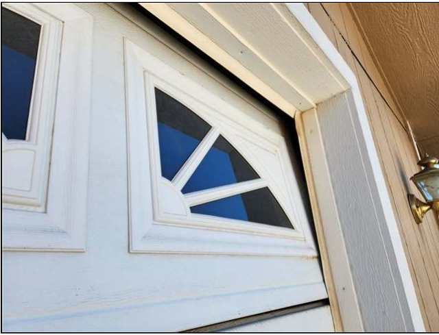
11.2 Item 1(Picture) Garage door is NOT fully installed
