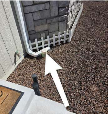
Drain, Waste, & Vent Systems: Sewer Cleanout Location
