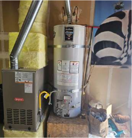
Hot Water Systems: Location Garage
