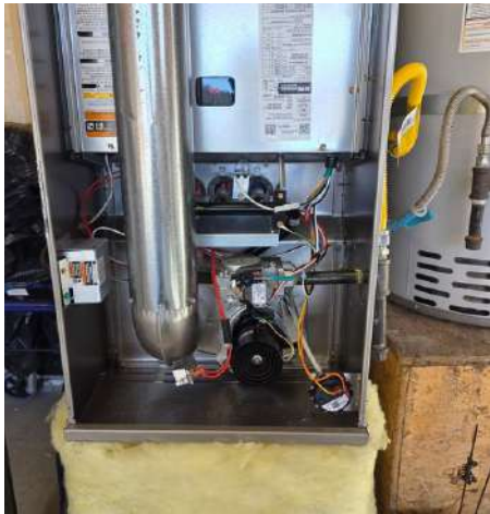
Equipment: Brand Bryant
