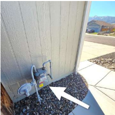
Gas Distribution System: Main Gas Shut-off Location Gas Meter, Front, Left
